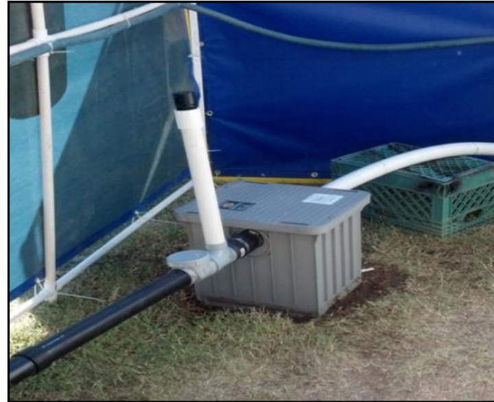
Wastewater Connection with Grease Trap
